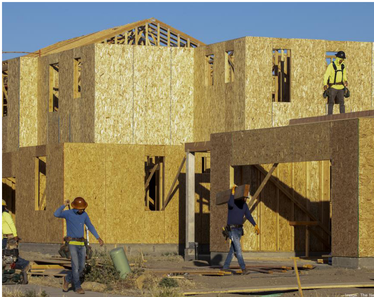
Construction on a home in the River Islands subdivision in Lathrop, California, May 5, 2021. Last year, California issued about the same number of permits for single-family homes as the Houston metro area.
